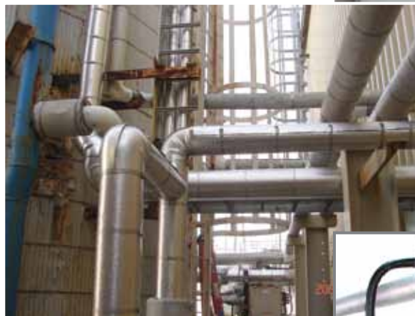
Completed piping project at a combined cycle power plant—electric heat trace with insulation.
