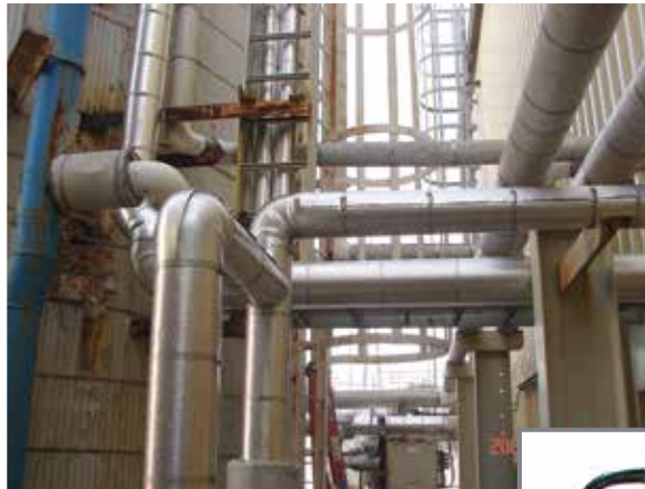
Completed piping project at a combined cycle power plant—electric heat trace with insulation.
